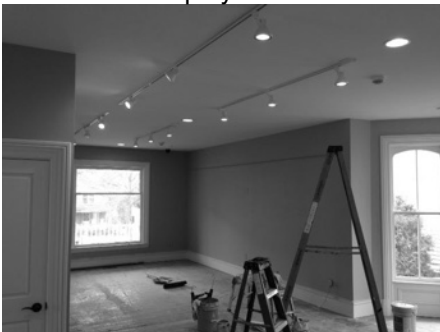
Track lighting in front room display area
